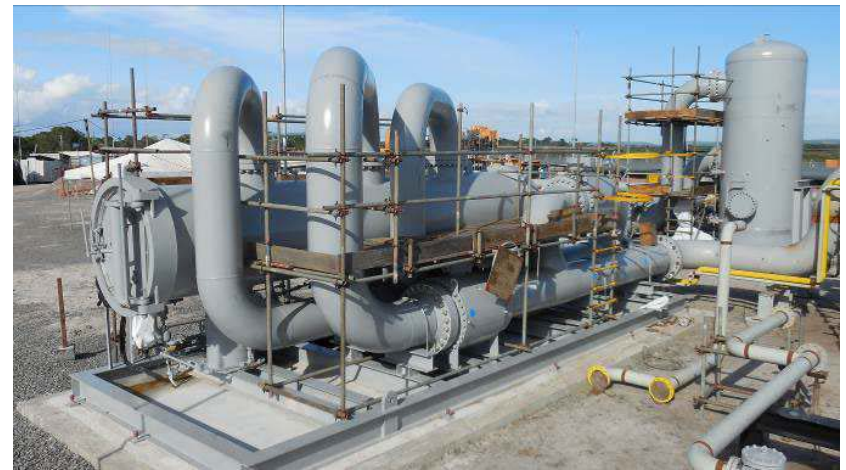
Detail of one of the compressor skids
