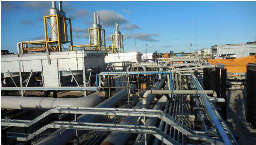
Overview of the Compression Plant of the Manati Field
