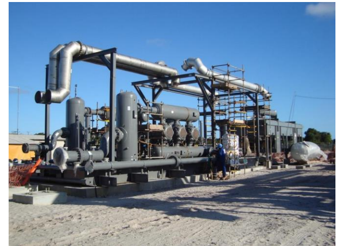
Detail of the compressor
