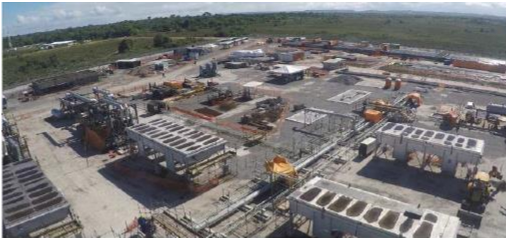
Overview of the Compression Plant of the Manati Field
